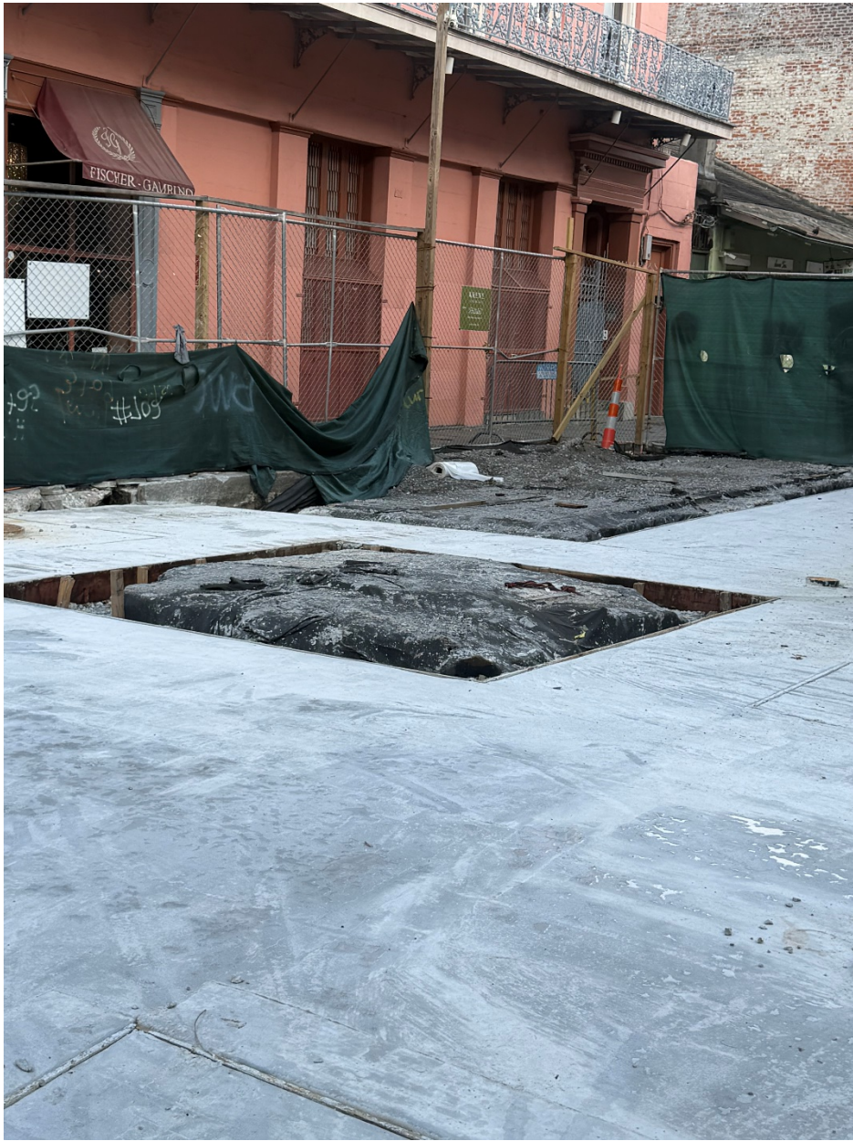
St. Peter & Royal Street areas waiting for Entergy Electric
